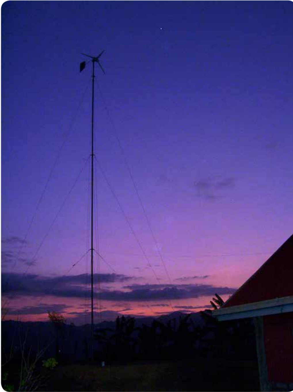
Lamag Wind Turbine, Ilocos Sur.
