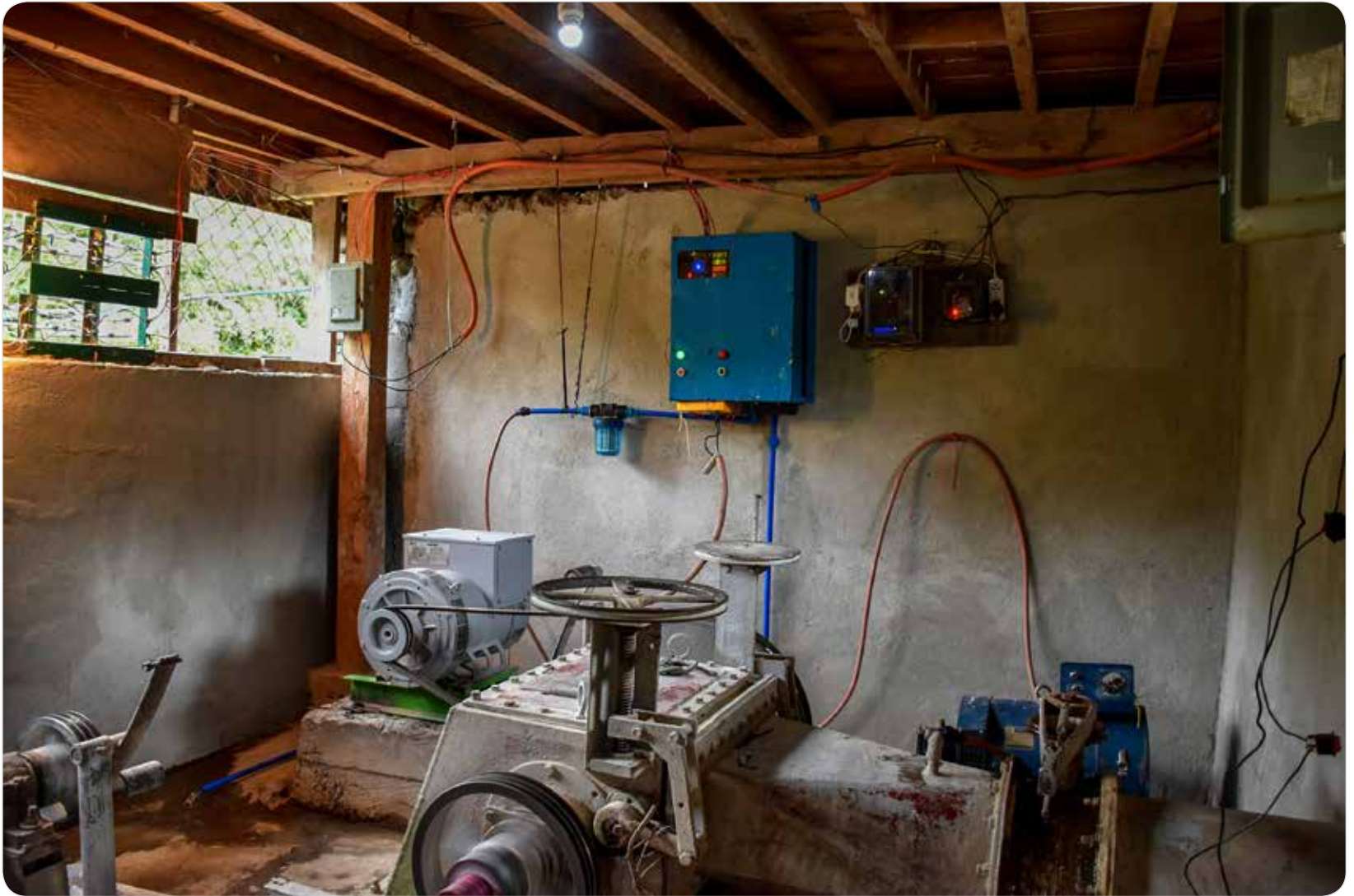
The powerhouse houses the electromechanical parts of the microhydro, comprised by the turbine, generator and load control.
