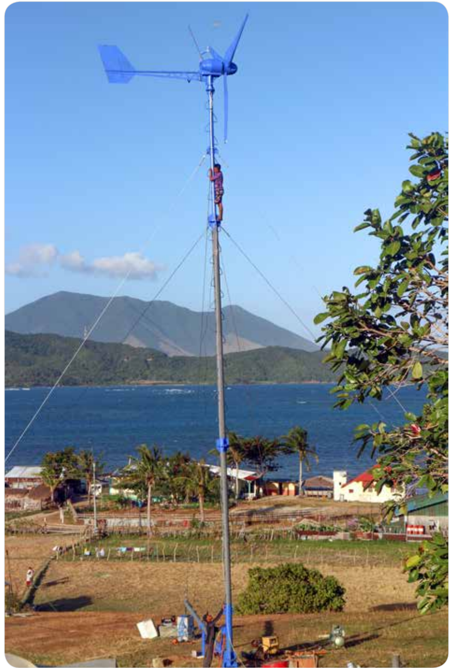
The 2-kW hybrid wind-solar system for water supply in Brgy. Bonbon, Municipality of Looc, Lubang Island, Occidental Mindoro.
