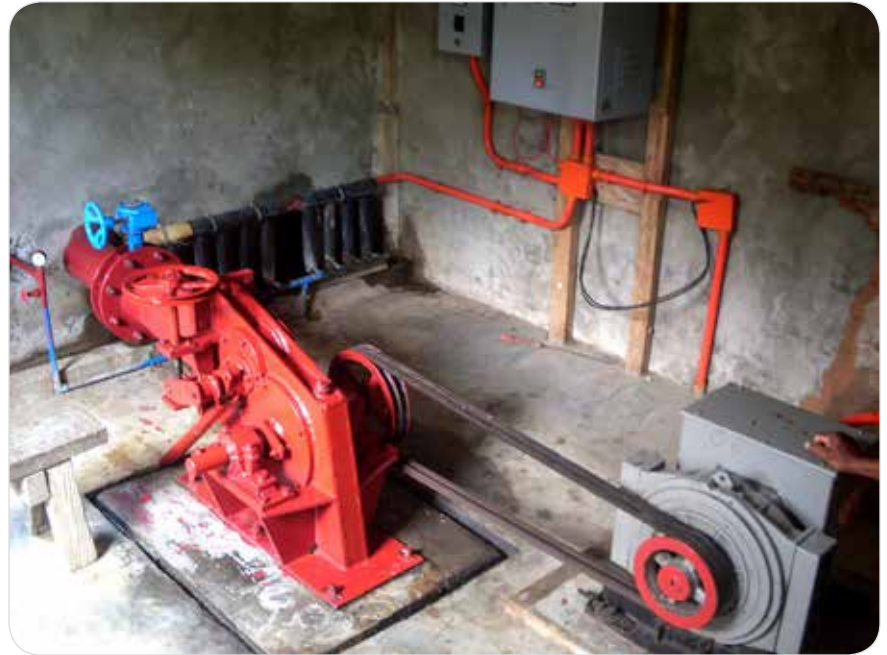
Crossflow turbine of the Lapat-Nanawatan microhydro.
